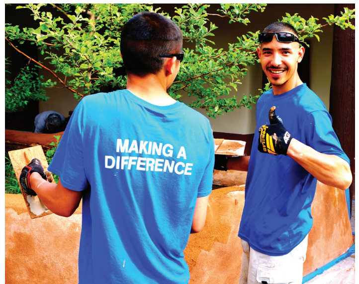
Alex Rendon and Michael Gonzales working on historic preservation of Santa Fe Trails building.
